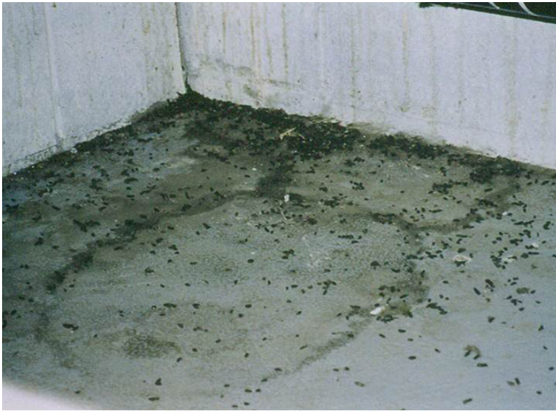
Photo 3 - This mechanical room which doubles as a return air plenum shows evidence of moisture entry from the adjacent outdoor air intake. It is also contaminated with organic matter.
