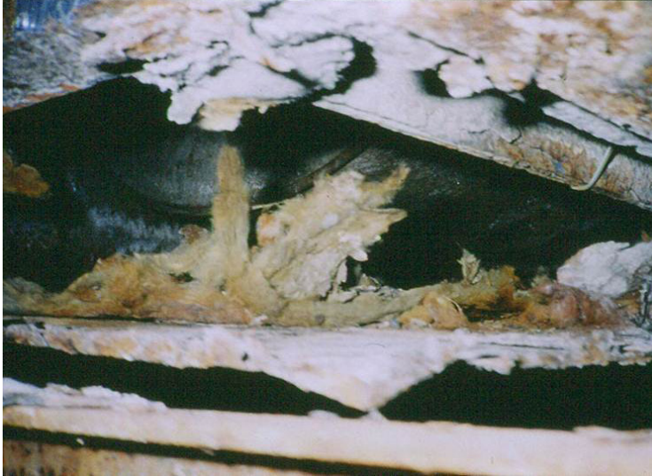
Photo 5 - The bottom of this fan cabinet rusted through because of a humidifier leak.
