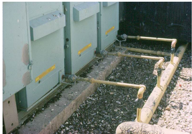
Photo 2 - Ballast near this air intake makes removal of bird droppings difficult
