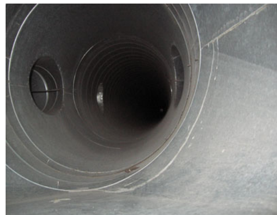
Photo 6 - Air duct after cleaning
