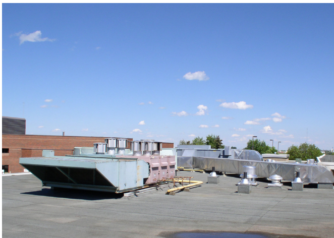
Photo 1 - Roofs can be crowded spaces with air intakes next to vent stacks
